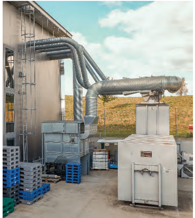
The suction plant in the BOBST Competence Center operates with an air volume flow of 24,000 cubic metres an hour.
