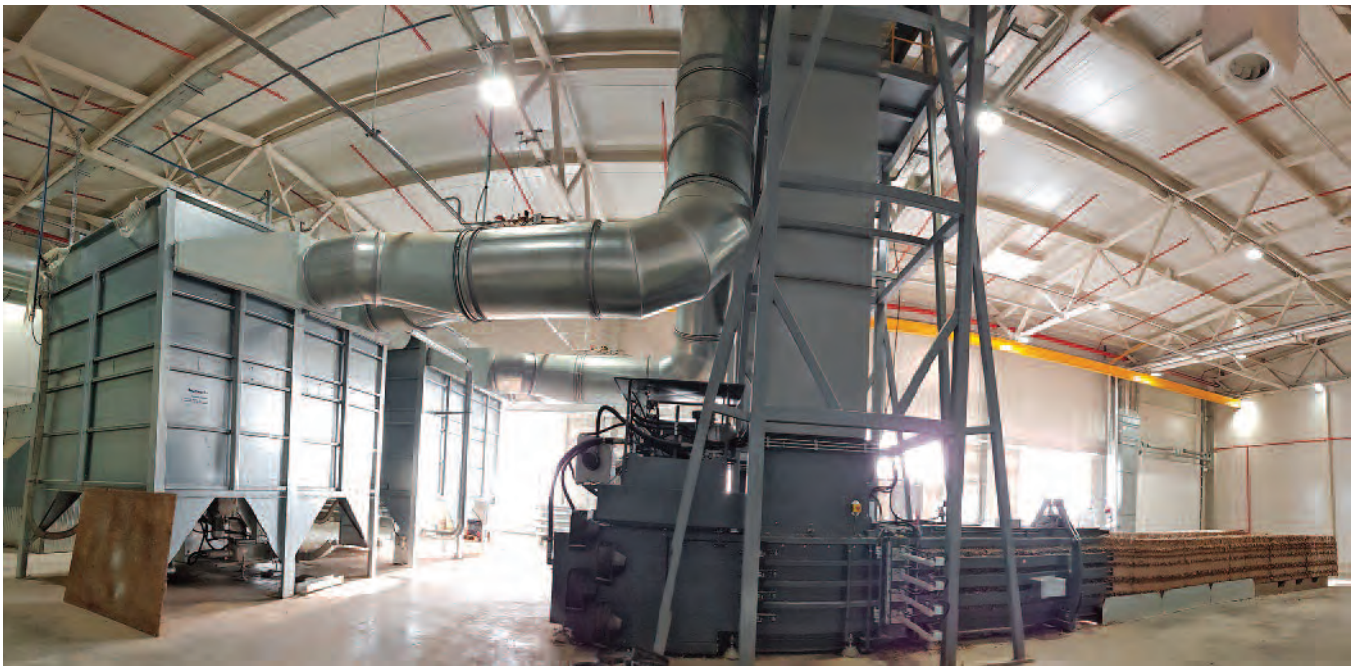
To ensure that the great quantity of cardboard waste is reliably disposed of in 24/7 operation, Hunkeler Systeme AG installed two high performance baling presses from the series VK 4212. The cardboard waste is transported to the presses via paper cutters.
