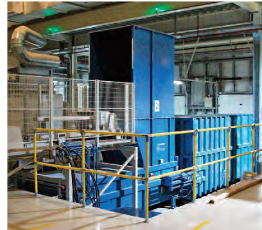
Ten containers serve seven stationary presses. This ensures that both production and the filling of the containers with the waste material is a nonstop operation.
